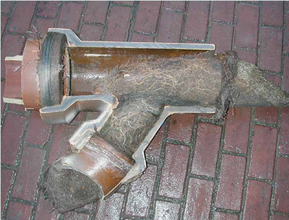
Root intrusion into private sewer laterals
