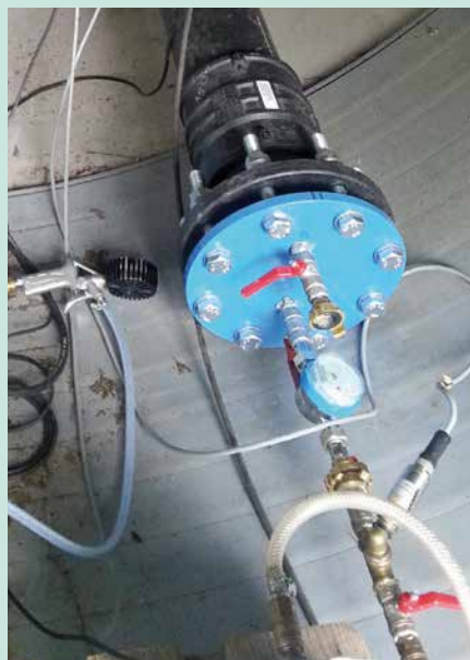
IKT technology in use: a pressure sensor in the supply line
