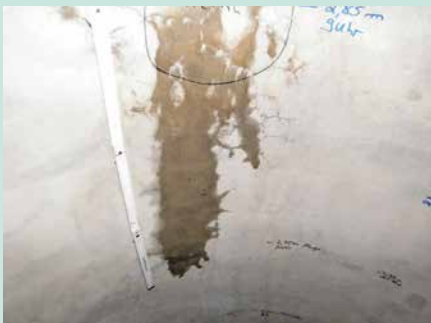
Damp patch with spreading plume
