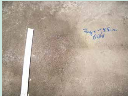
Damp patch larger than 25 cm
