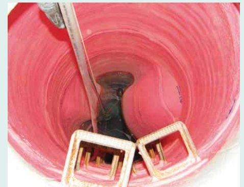
System failure: It was not possible to evaluate the „Spectrashield“ system.
