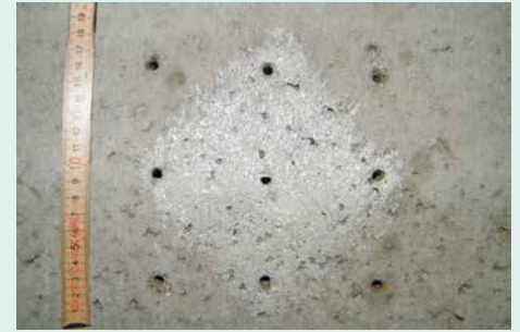
Area damage: nine drilled holes of 5 mm dia. in an area of 20 x 20 cm and application of mould release agent to a small area
