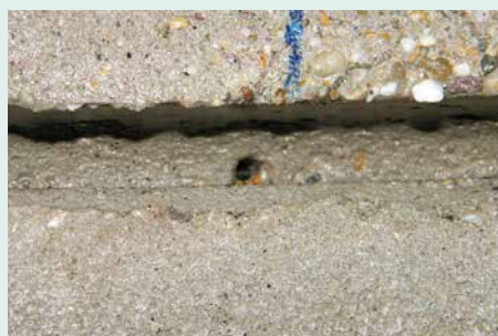
Five leaking ring joints per manhole: four drilled holes of 6 mm dia. per joint
