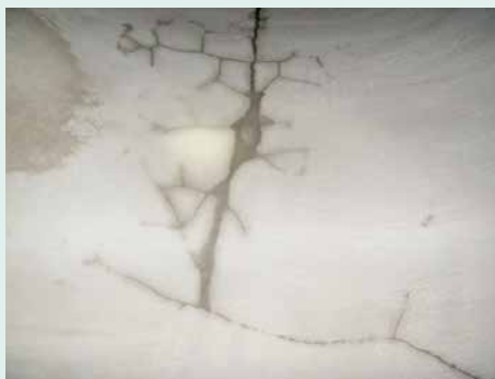
Cracks are indicative of an inadequate adhesive bond with the substrate.
