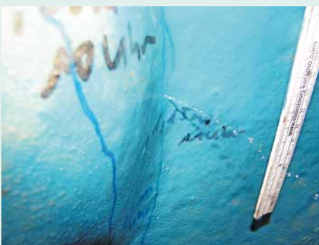
Deficiencies in substrate preparation: blisters and cracks may be the result if the mould release agent prevents secure bonding.
