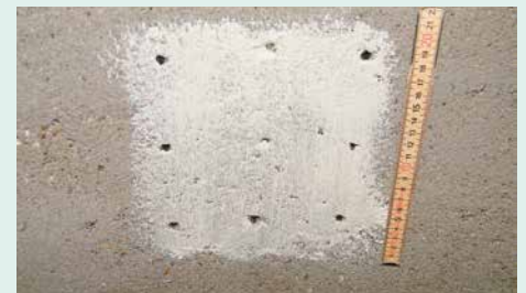
Area damage: nine drilled holes of 5 mm dia. in an area of 20 x 20 cm, application of mould release agent to a large area
