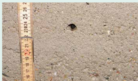
Isolated damage: every manhole was subjected to „pre-damage“ in the form of eight drilled holes (dia.: 10 mm).
