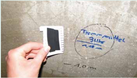
Cracking in a zone pre-treated with mould release agent.
