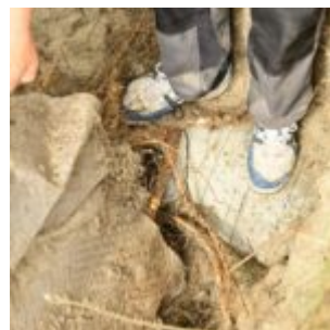
Protective mat, roots and sewage pipe
