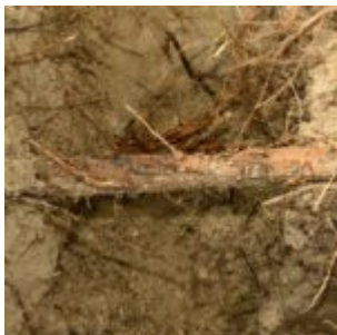
Horizontal root ingrowth in the pipe trench
