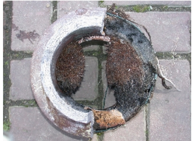
Pipe joint exhibiting severe root infiltration
