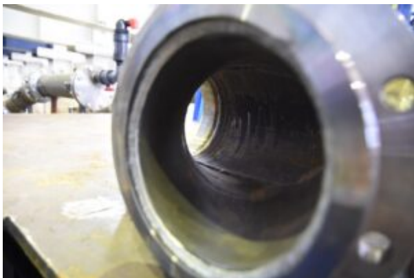
30° bend in a pressure sewer pipeline
