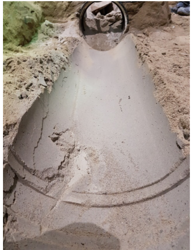
Pipe enclosure with minor defects (DN 300)
