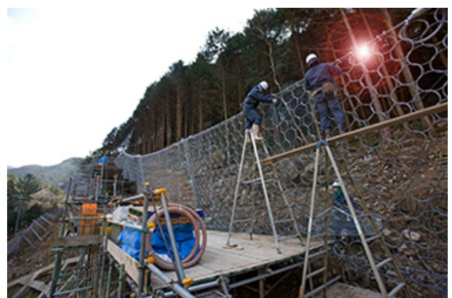
High tensile steel mesh barrier for rockfall
